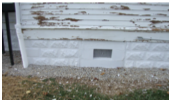
HUMC 'before' re-painting and 'after' foundation changes (window vent addition, painting) and drainage improvements.
